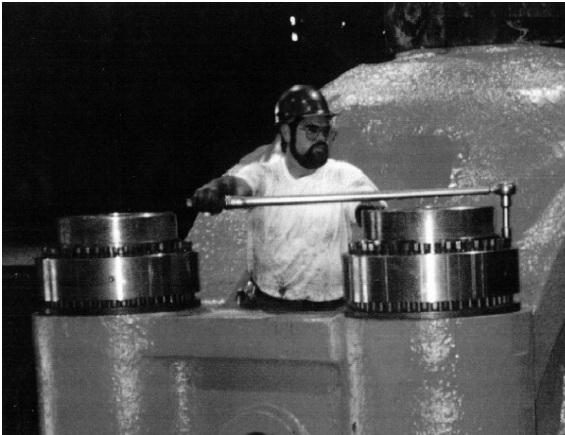
Figure 8. A worker torquing a SUPERBOLT® thrust collar assembly to tension an 18-inch (457.2-mm) tie-rod to a preload of 2,625,000 pounds (11,676 kN). The jackbolt torque being applied with a torque wrench is 275 foot pounds (372.9 NM) SUPERBOLT® Inc.
